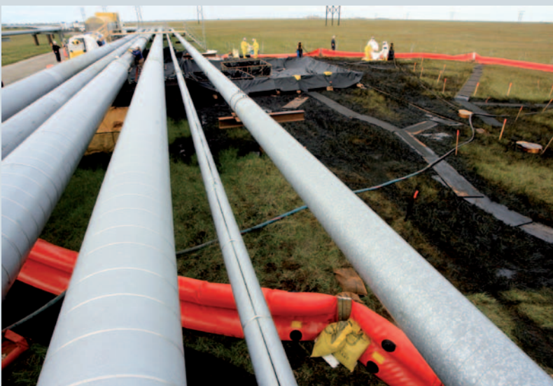
FIGURE 1: Cleanup and repair work after a pipeline leak (source: © ddpimages /AP Photo/Al Grillo)
